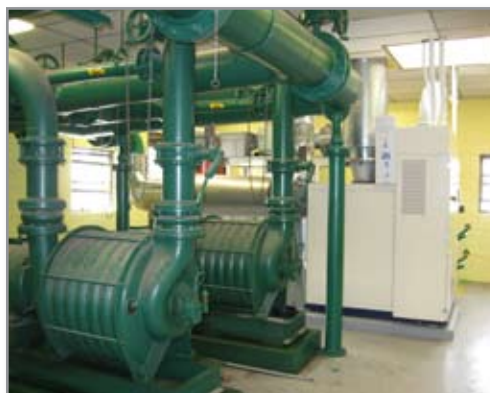
Existing Multi Stage Centrifugal Blower in Foreground with New Single Stage Centrifugal Blower
